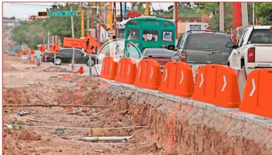
Dry box of 53" with approx. 1,134 nestable barriers. Channelizing 5,580 linear ft.
